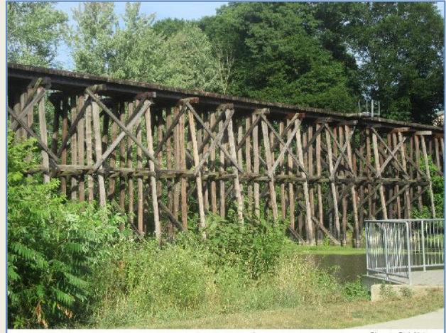
Railroad Trestle in Hamilton, MI Built 1868-9 first used in 1870. In service as of May 2022 under CSX. Photo by Rich Mahaney
