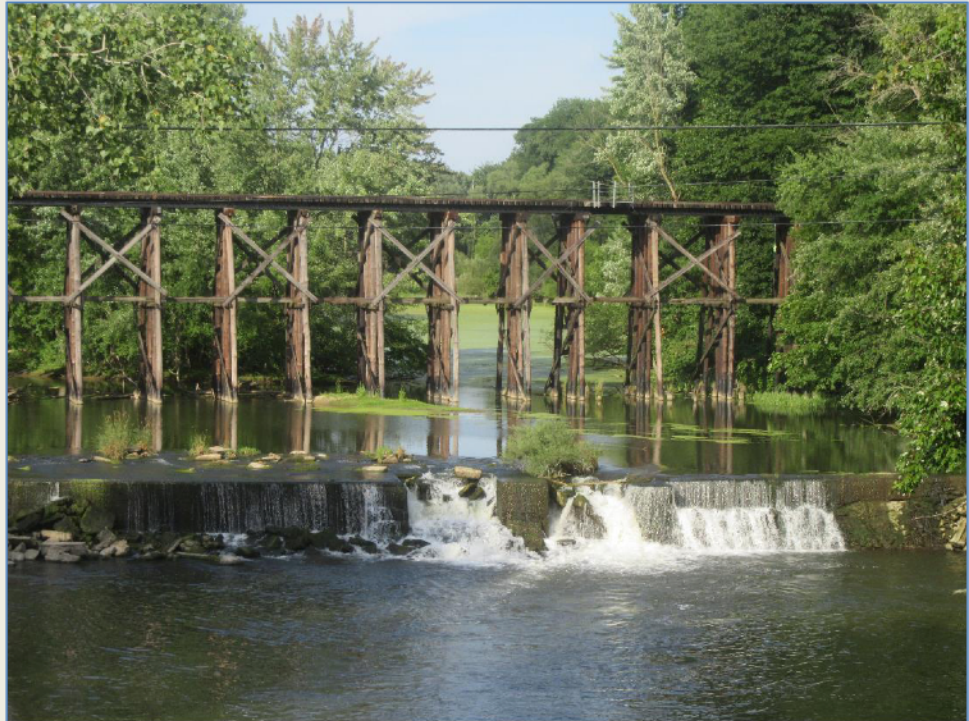
Railroad Trestle in Hamilton, MI Built 1868-9 first used in 1870. In service as of May 2022 under CSX. Photo by Rich Mahaney
